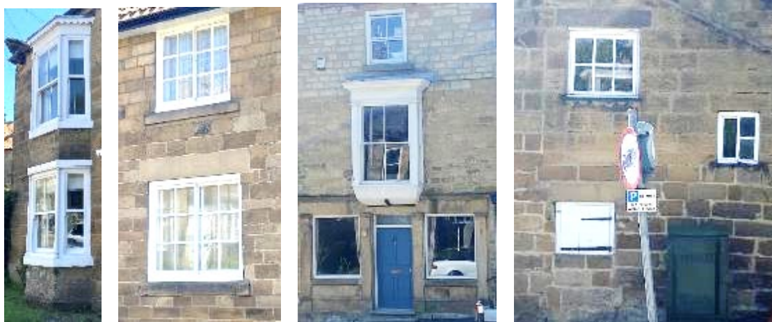
Figures 62-70: Window types in Osmotherley including the Yorkshire sliding sash; tripartite Yorkshire sliding sash, 8/8 sliding sash (there are good examples of 6/6 sliding sashes in the village too) and the Victorian 2/2 sliding sash.
