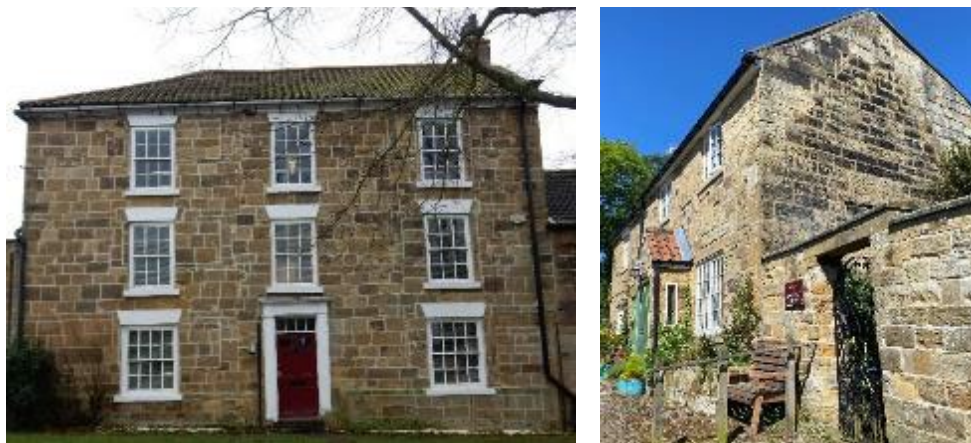
Figures 49-50: A extensively reworked façade and evidence of a previous steeply pitched thatched roof.
